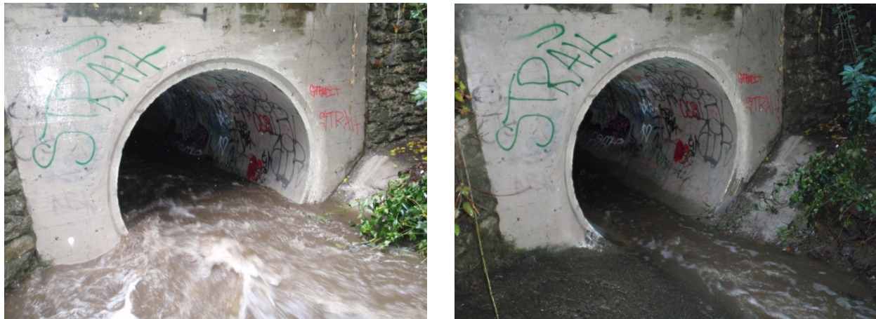
Figure 32: The photo on the left shows the October 19, 2009 peak discharge water surface elevation at the upstream end of the culvert at El Centro Avenue. For comparison, the photo on the right shows conditions during low or base flow.
