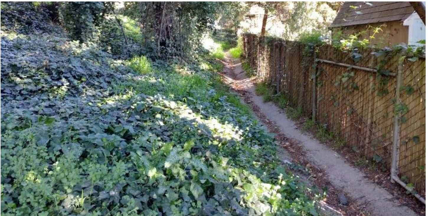
Figure 4: Concrete swale running above the culverted section of Sausal Creek within Wood Park
